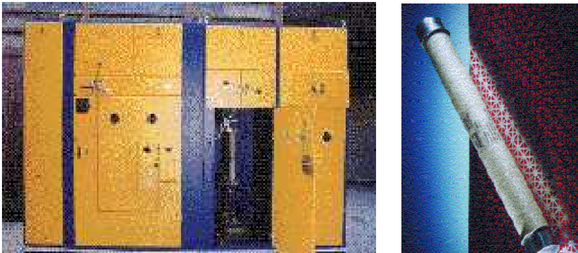
Figure 3: indoor type fuses installed in the primary of the transformer
